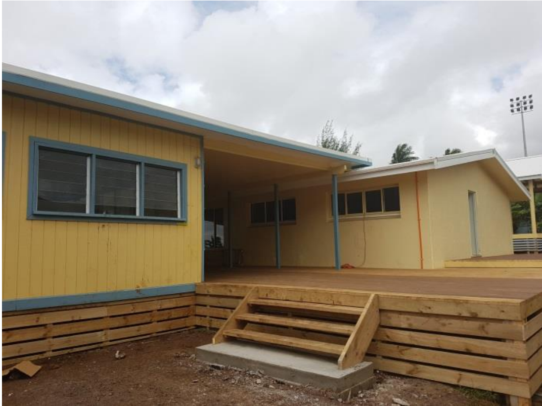
Relocated Food Technology building connected to Maori and Cultures classroom by an outdoor learning area.
