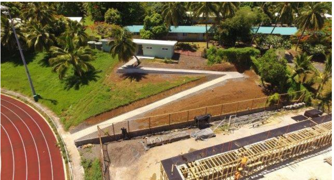
New walkway on the southern bank of the BCI Stadium that will provide safe access between the upper and lower quads during the construction period.
