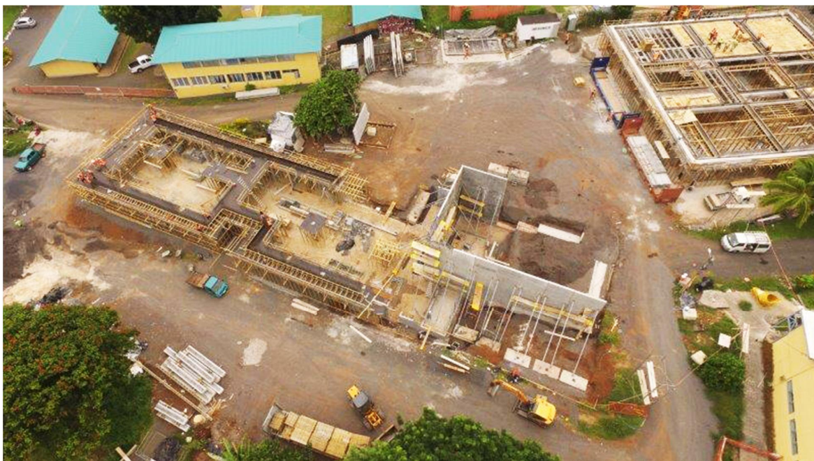
All precast beams have been landed and all precast panels have been fabricated. A number of precast panels – including those indented with Polynesian motifs – have been mounted at the Seminar room. Image taken Tuesday 11 th April.
