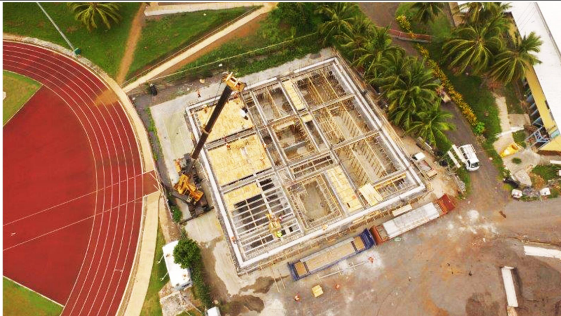
Stahlton's Rib and In-fill flooring system arrived last week, initiating work on the first floor of the Technologies building. Image taken Tuesday 11 th April 2017.
