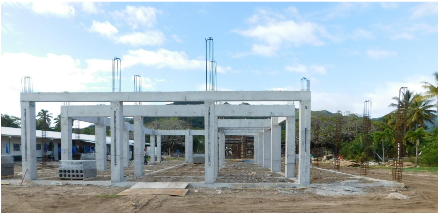
Formwork at the ECE building has been removed and contractors are now in the process of completing the steel and form work for the structural elements in the main building and senior school.
