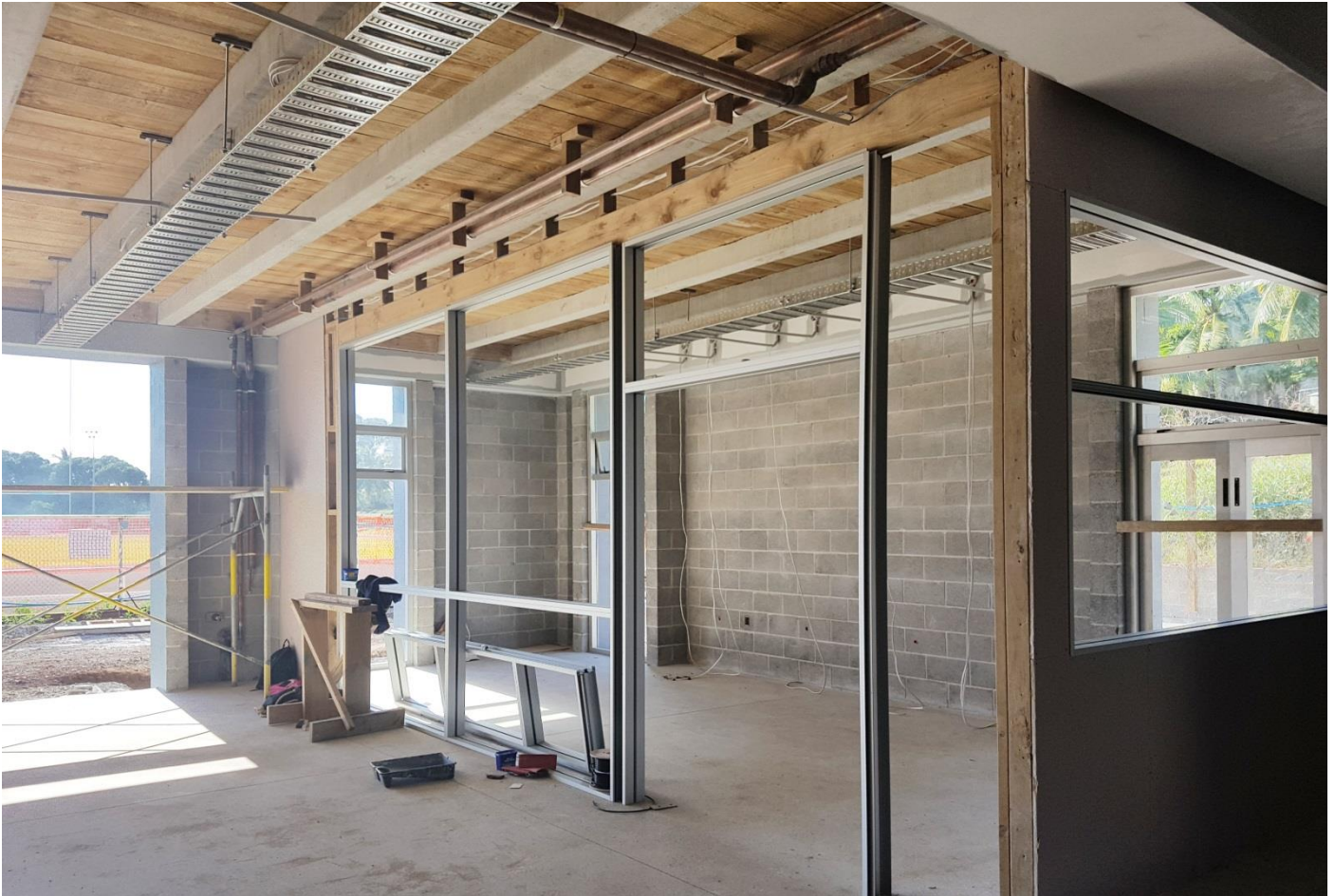
Technologies Building (Construction and Mechanics room): More than 80% of the aluminium window and door frames have been installed.
