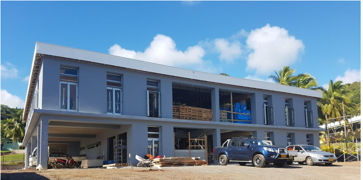
Technologies Building: Waterproofing and painting of the exterior block work is complete and contractors have begun to paint the internal spaces.
