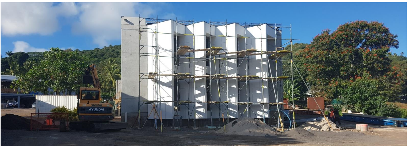
Student Research/Admin Building: All roofing iron has been placed, and the gutter system is 95% complete.
