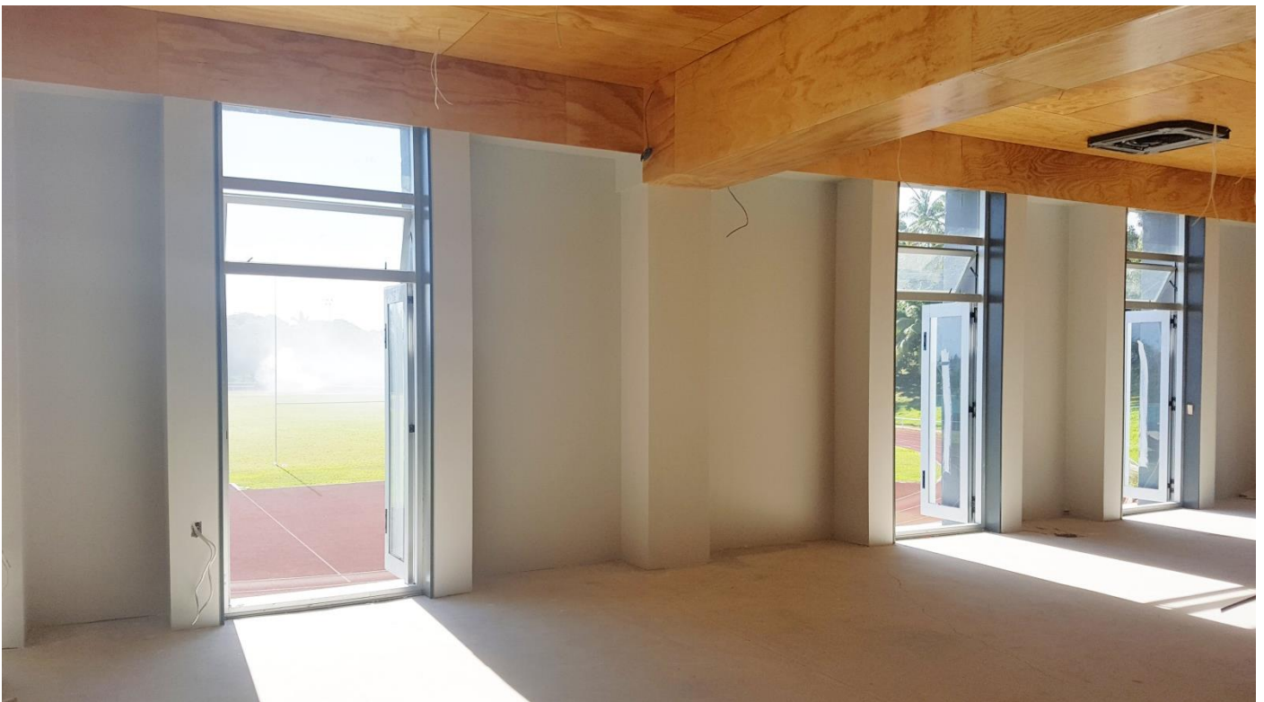
Technologies Building: Lining of internal walls and ceilings are well underway and contractors have begun to paint the internal learning areas.
