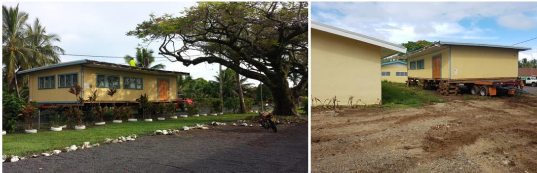
Left: Food Technology building being moved by Multicontractors Ltd. Right: Building positioned adjacent the refurbished house on the east boundary.
