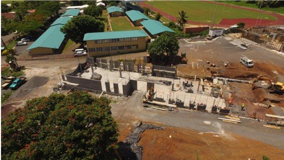
Student Research Centre and Administration building: 80% of the ground floor and 25% of the exterior block work is complete
