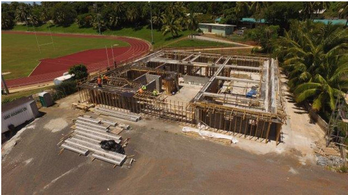
Technologies Centre: 90% of the ground floor slab and 50% of the exterior block work is complete. Construction of formwork for the first floor slab continues.
