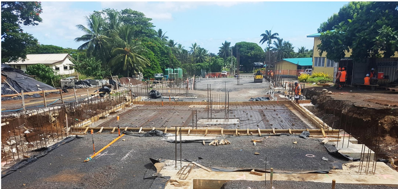
Student Research Centre and Administration building – Building footprint has been backfilled and compacted. A section of the ground floor has been boxed in preparation for the slab pour.
